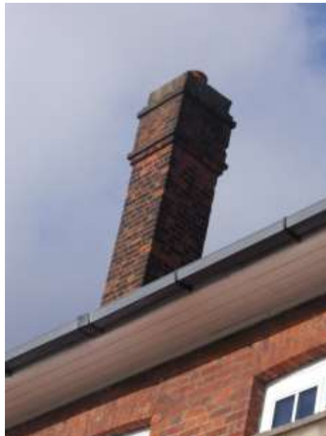
Figure 71: Tall chimneys to the fire station form part of its Arts and Crafts character
